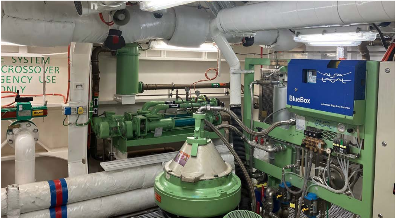
The vessel's oily water separator is monitored by video surveillance in the engine control room. MARINE EXCHANGE OF ALASKA
