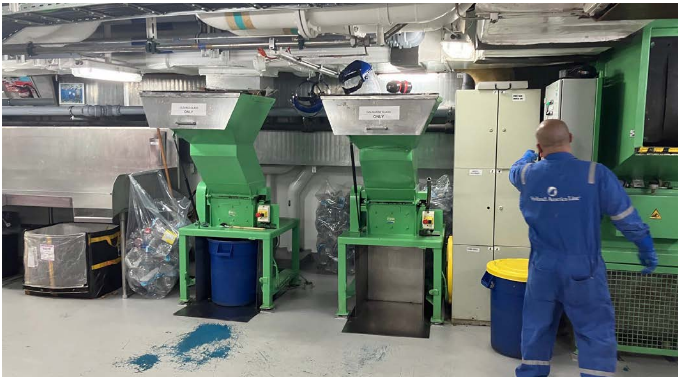
Cruise ships closely manage recyclables, non-recyclables, food waste, and other components of waste management in the waste sorting and handling room. MARINE EXCHANGE OF ALASKA
