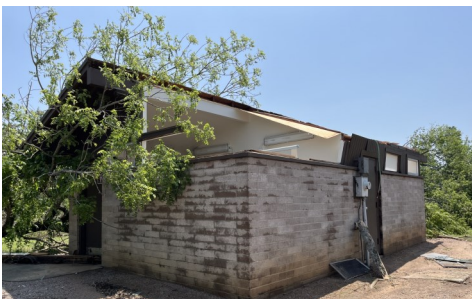
Tornado damage at Chickasaw National Recreation Area © NPS
