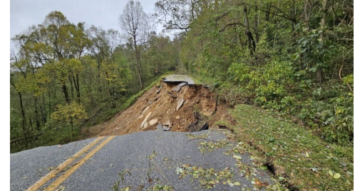
Collapsed roadbed at Gooch Gap, Blue Ridge Parkway © NPS
